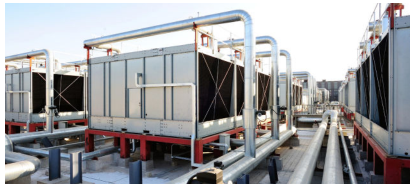
Sets of cooling towers atop a data center facility
