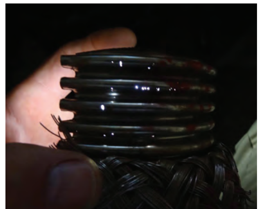
Flashlight reveals pinholes caused by pitting corrosion
