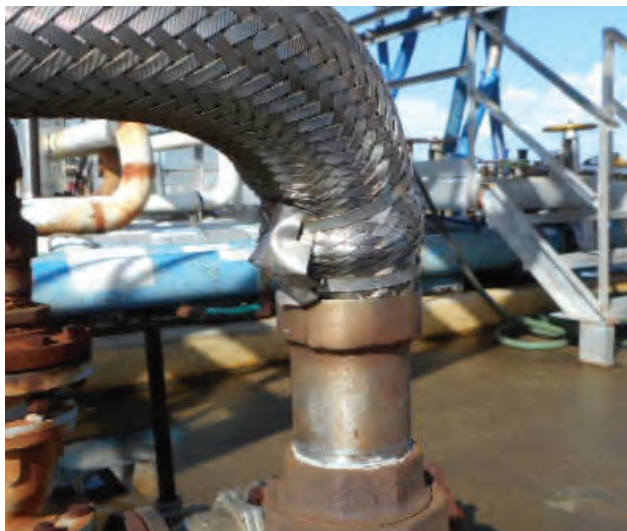
Extreme overbending on a terminal dock
